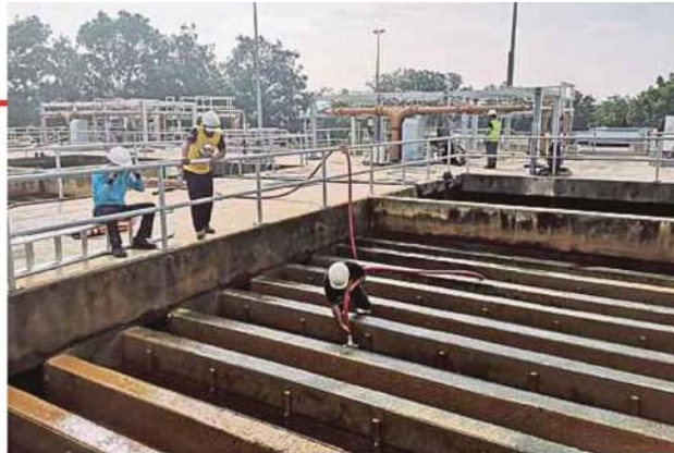
Upgrading work being done at the Sungai Selangor Phase 2 Water Treatment Plant on Wednesday.
